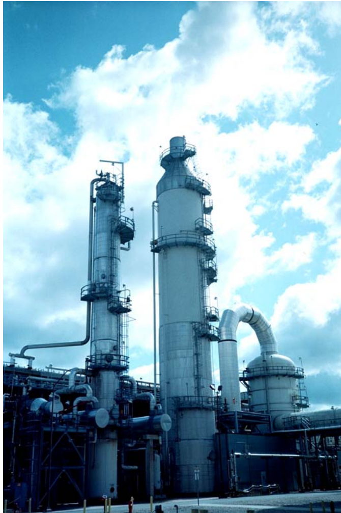
Figure 3: Bellingham Econamine FG SM Plant Ground View
